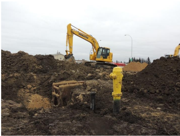
Fire Hydrant at RM West Service Road 2016
