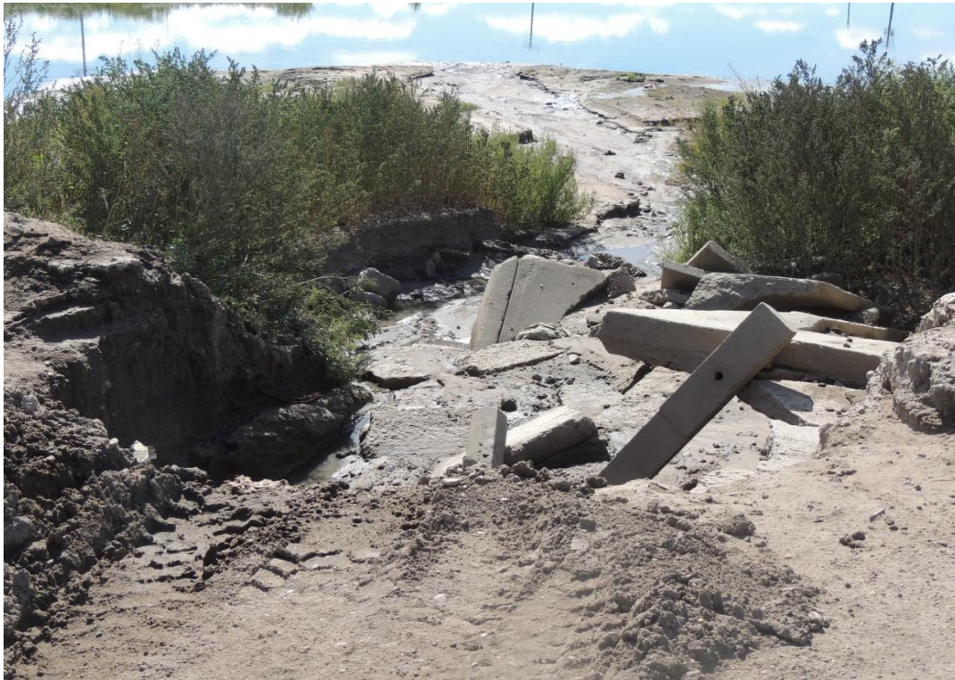
2016 Eroded Dump Chute
