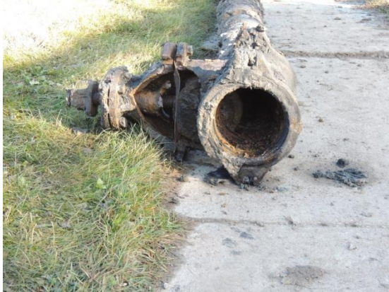
Valve Removed 6 th Ave W and 3 rd St. W
