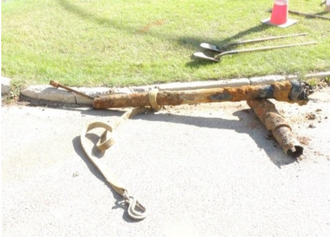
Typical Valve Box Removed, Corroded, Segmented, Filled With Sand – 2016
