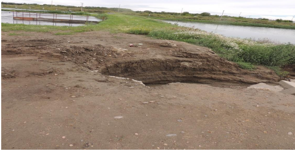
2016 Eroded Dump Chute
